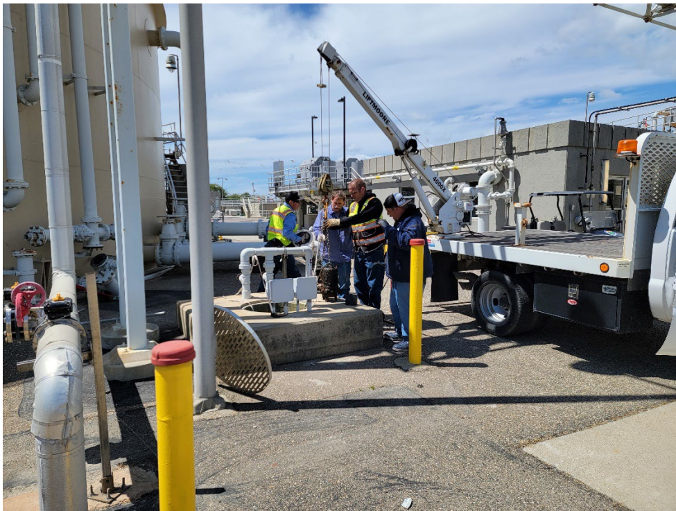
Senior Operator Rick Jackman, Operators Justin Musick and Mario De Leon, and Operator in Training Everardo Vargas performing the removal of a sump pump.
