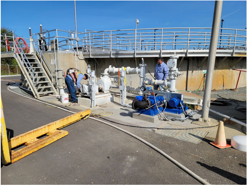
Operator Justin Musick and Operations Supervisor Mike Arias installing new PC2 Sludge Pump.
