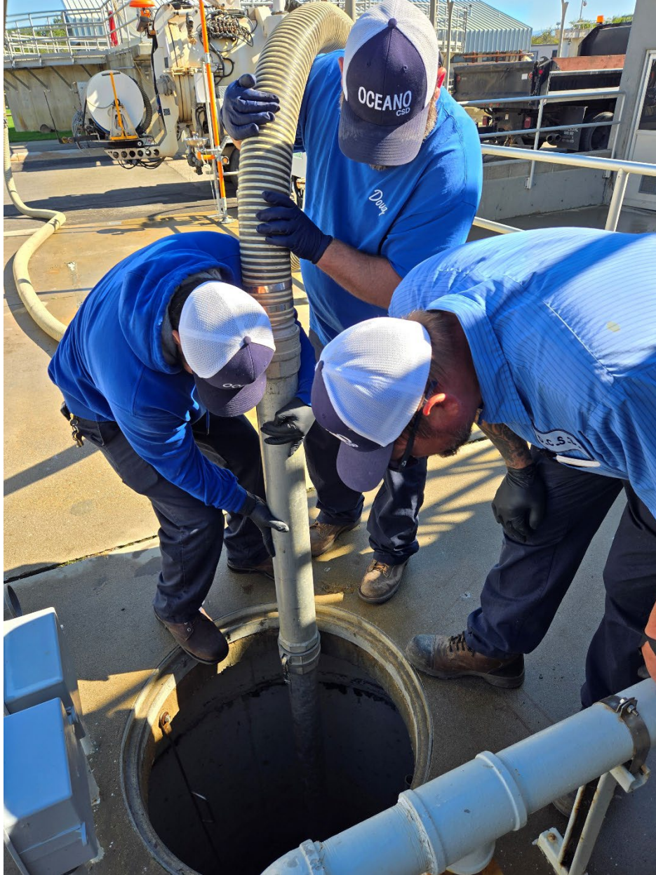
Oceano Community Services District Staff performing vacuum truck services on a sump at the District treatment facility.
