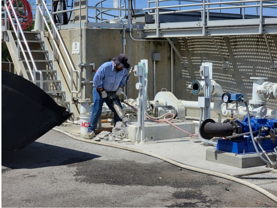
Operator in Training Robert Grajeda performing demo of the old PC2 sludge pump.
