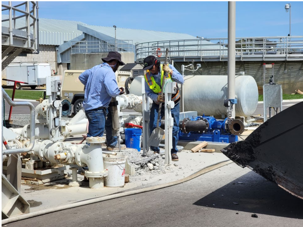
Operator in Training Robert Grajeda and Operator Justin Musick continuing demo of the old PC2 sludge pump.
