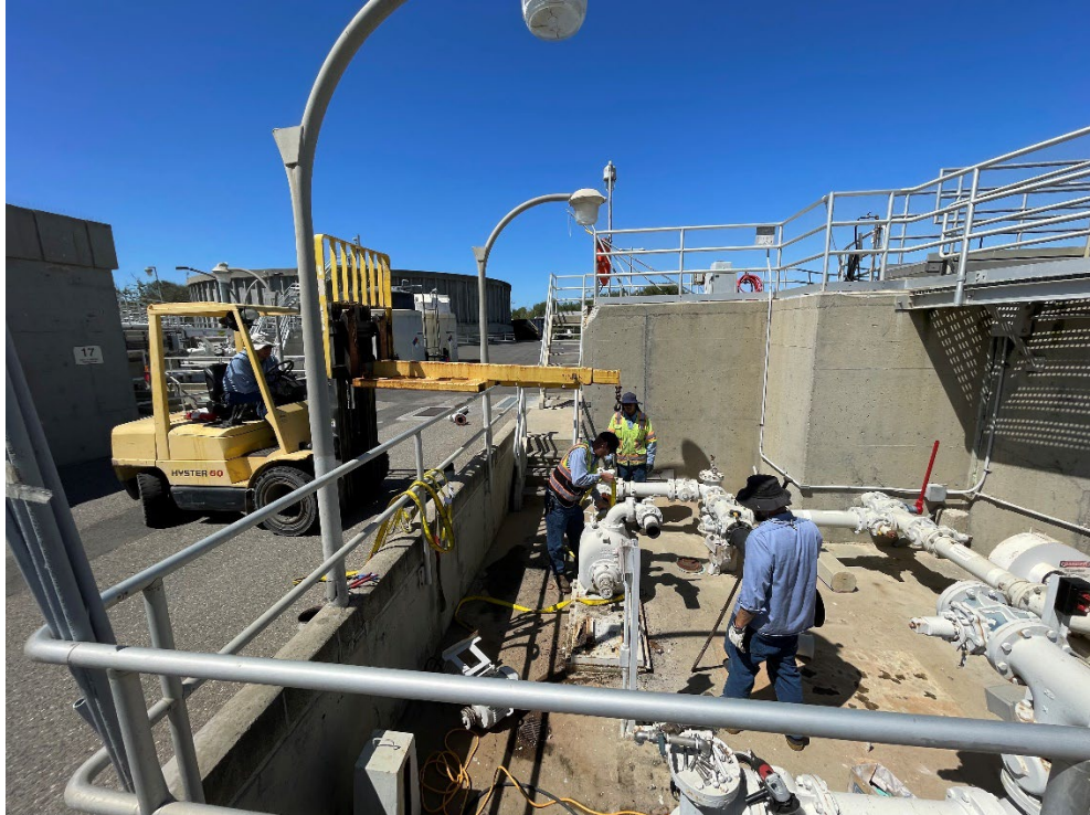
Operator in Training Everardo, Nick Kurokawa, Robert Grajeda, and Operator Justin Musick performing demo of the old PC1 sludge pump.
