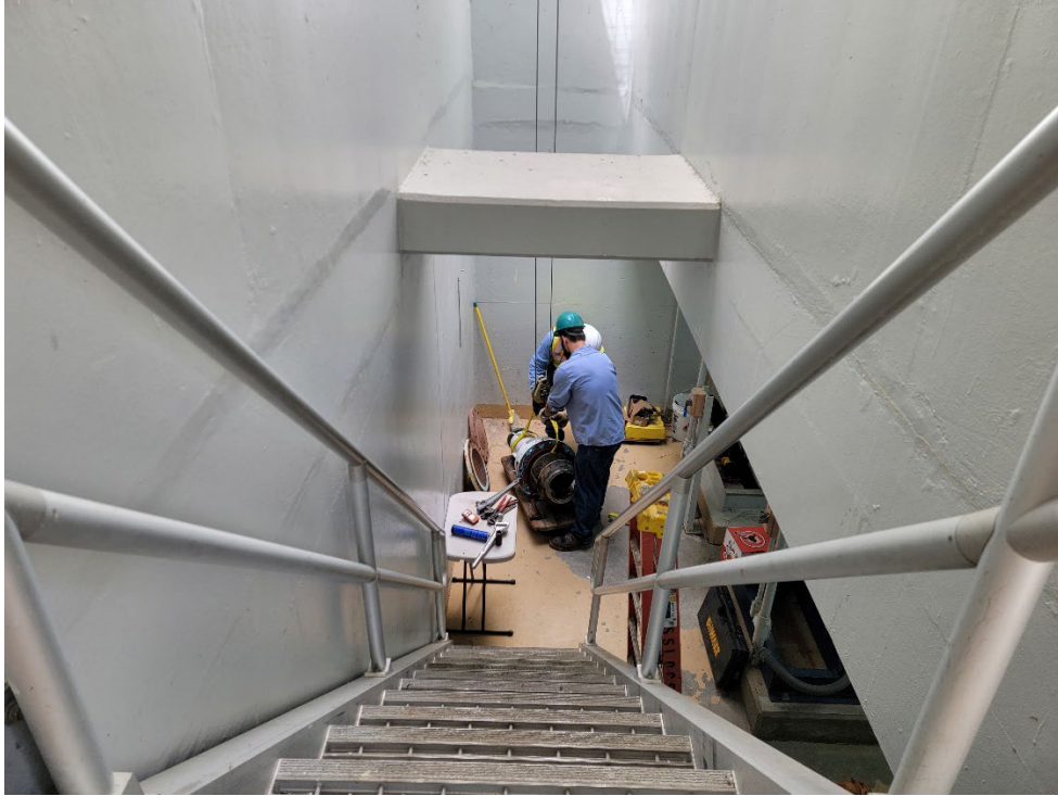
Operators in Training Robert Grajeda and Everardo Vargas preparing Influent Pump No. 3 for retrieval from the Influent Pump Room.
