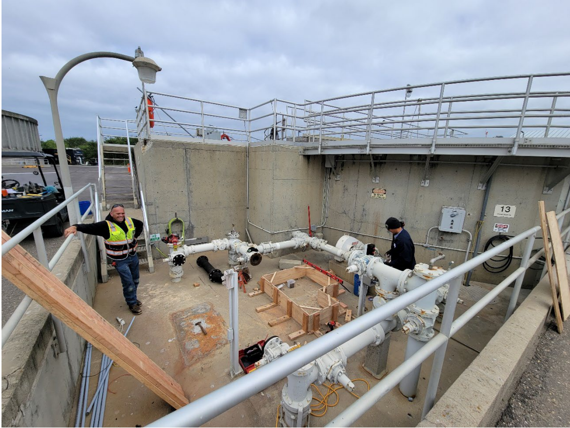
Operator Justin Musick and Operator in Training Nick Kurokawa installing forms for the new PC1 sludge pump base.
