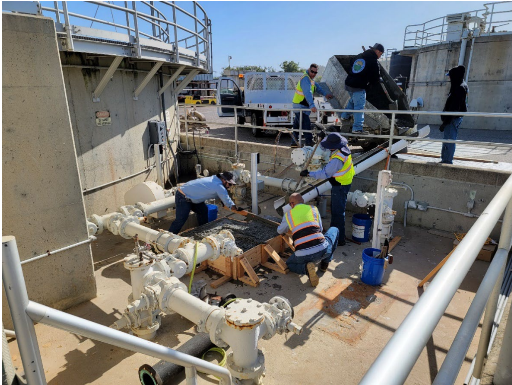
District Operators pouring new concrete slab for new Primary Clarifier No. 1 sludge pump.
