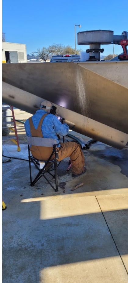
Brian Ventura from Ventura Welding performs installation of stainless-steel patch on District Grit King.
