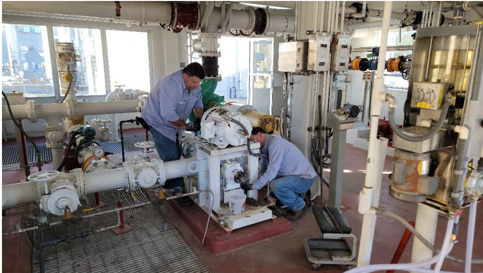
Operator Mike Arias and Rick Jackman performing the reinstallation of the sludge bed feed pump.
