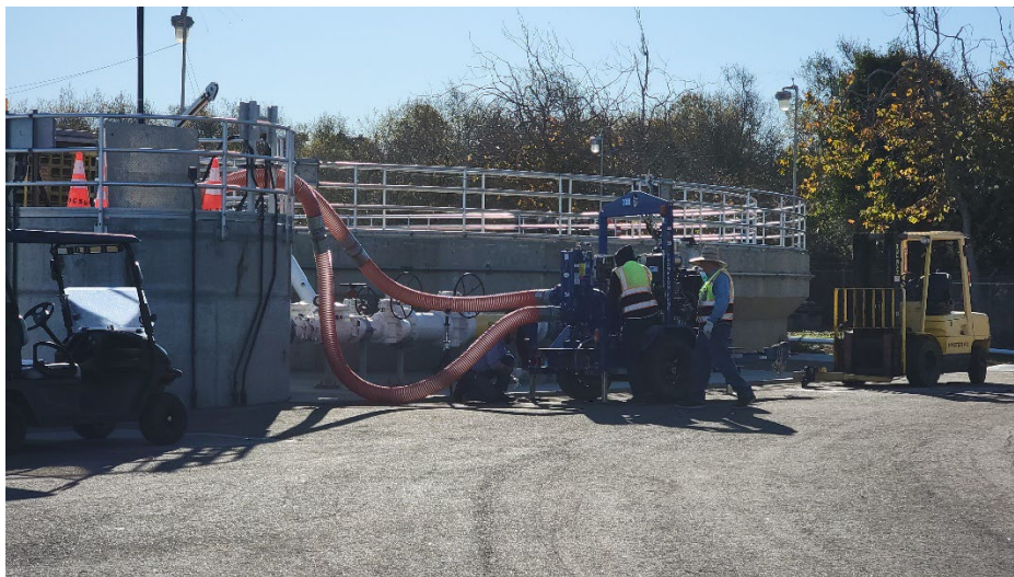
Operator Justin Musick and Everardo Vargas perform pump mixing of the SC1 Return Activated Sludge Well to breakup solids and surface scum.
