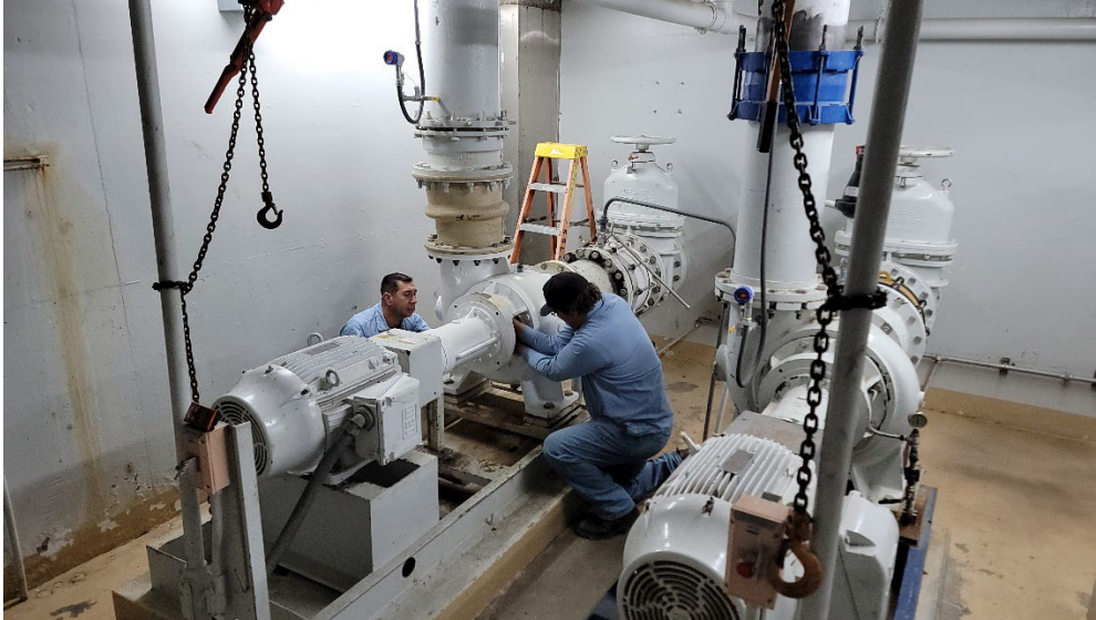
Operator Everardo Vargas and Chris Rigoni performing INF Pump No. 3 seal installation.
