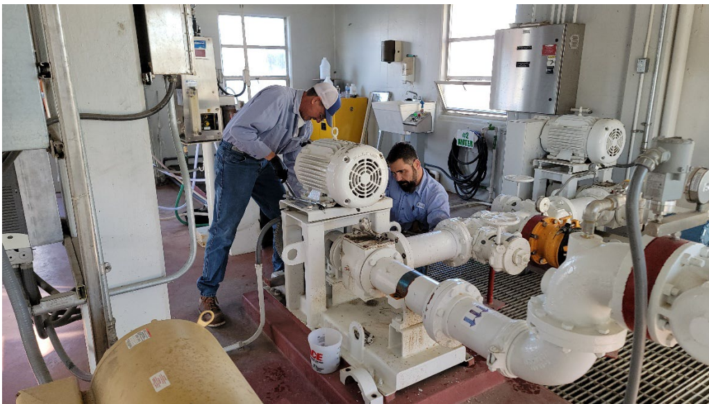
Operator Billy Romhild and Robert Grajeda performing the removal of the sludge bed feed pump.
