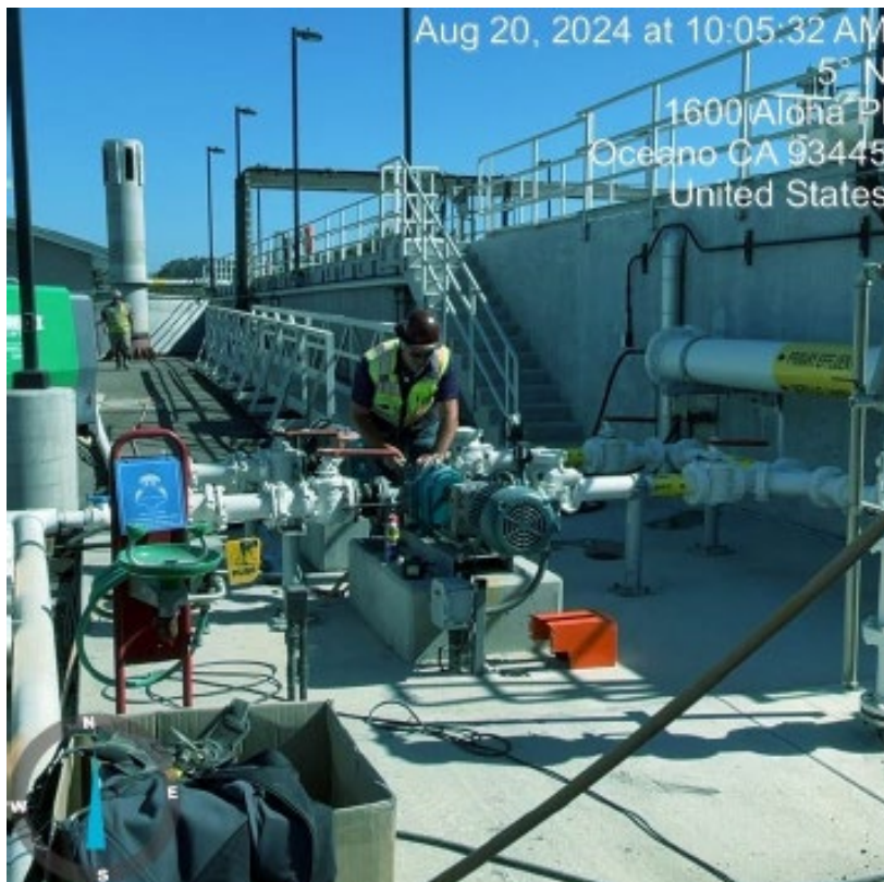
8.20.24 Servicing WAS Pumps
