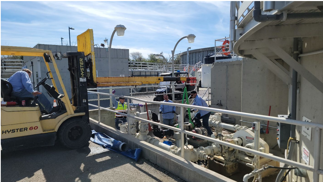
Senior Operator Rick Jackman along with Operators Everardo Vargas, Mario De Leon, and Justin Musick removing Primary Clarifier No. 1 sludge pump.
