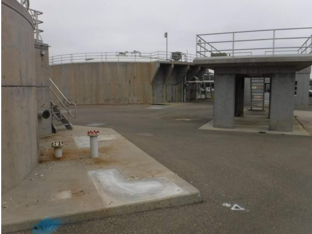
Photo 19 - East toward new Centrifuge
