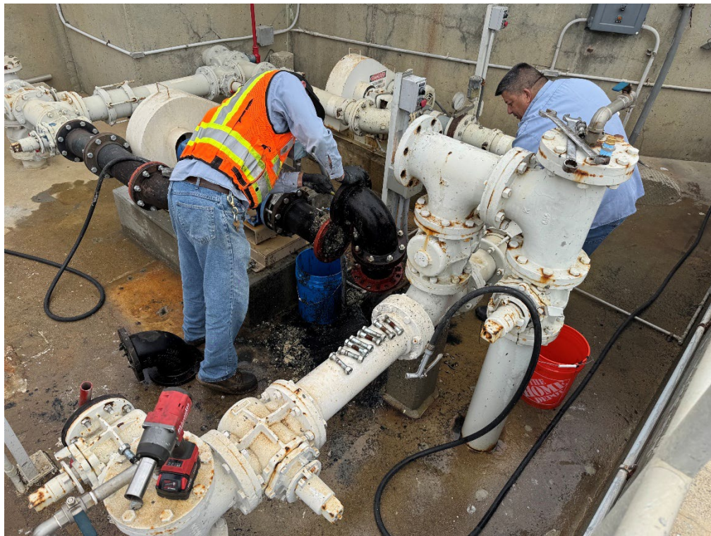
Operator Everardo Vargas and Operations Supervisor Mike Arias dismantling primary sludge pump No. 2 piping for inspection.
