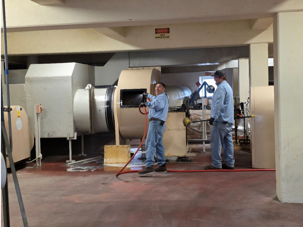
Operator Everardo Vargas and Senior Operator Christopher Rigoni performing preventative maintenance on the FFR supply fans.
