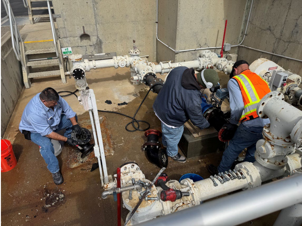
Operations Supervisor Mike Arias cleaning sludge pump piping while Operators Mario De Leon and Justin Musick reassemble cleaned sludge pump piping.
