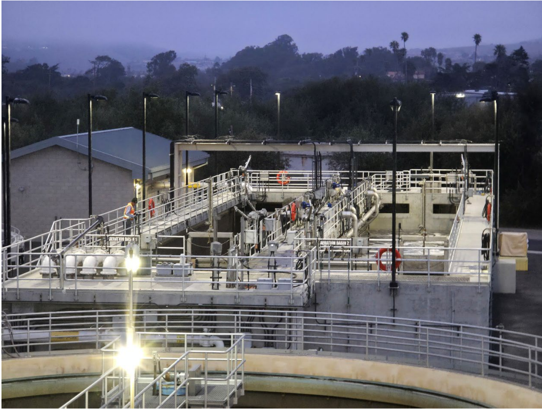
Operator Justin Musick monitoring the aeration basin process transfer.
